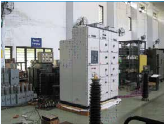
A view of 3 \Phi , 250kvar, 440 V, LV APFC panel undergoing tests
