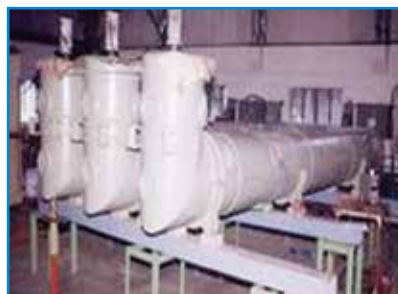
2. Isolated Phase Bus Duct
