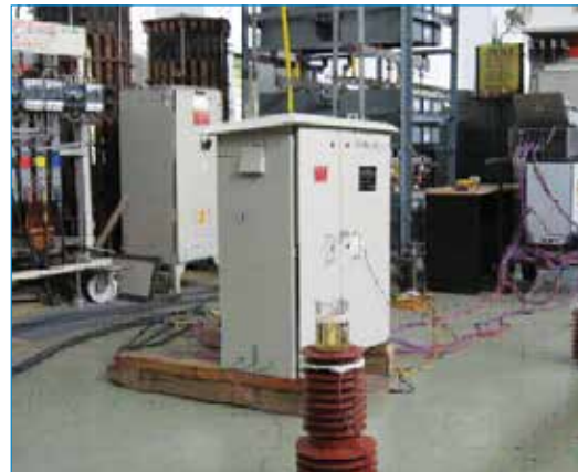
A view of the 3 \Phi , 100 kvar, 400 V, LV APFC panel undergoing tests
