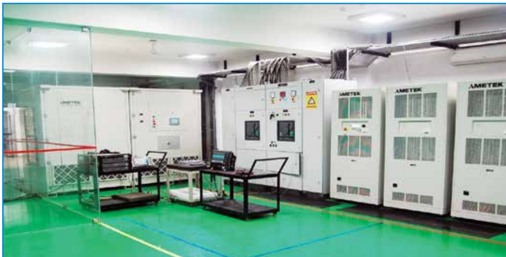
Grid tied inverter test facility
