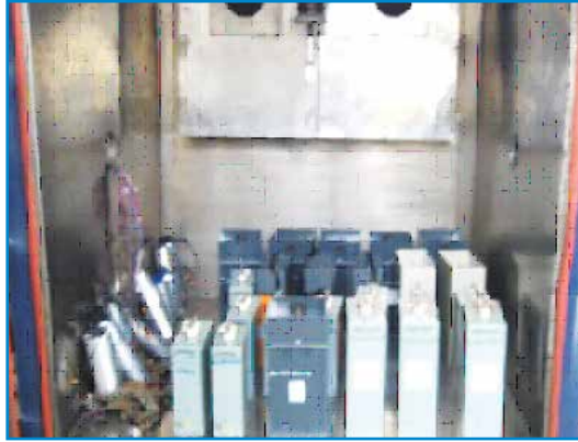
Some of the LV shunt capacitors tested
