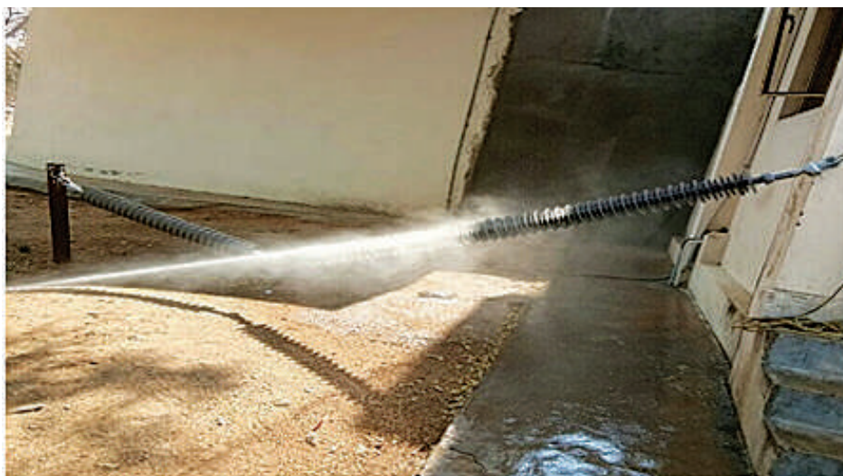
High pressure washing test facility for composite insulators at UHVRL-CPRI, Hyderabad
