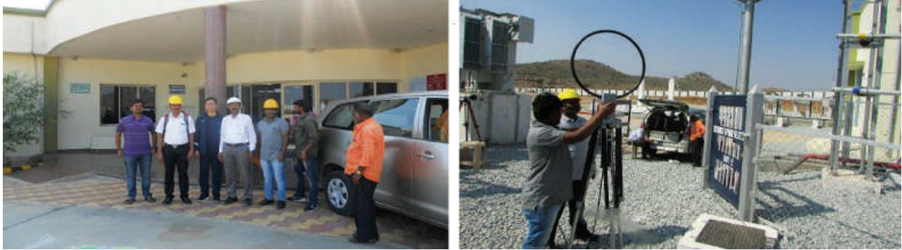
Measurement of Radio Interference Voltage (RIV) around 100 MVAR, STATCOM
