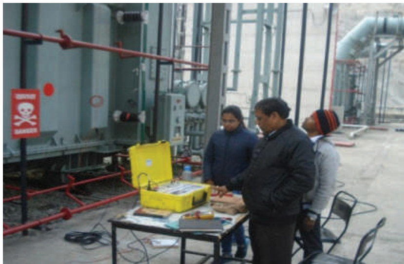
Diagnostic Testing on Generator Transformer at THDC India Ltd., Tehri Hydro Power Project Site
