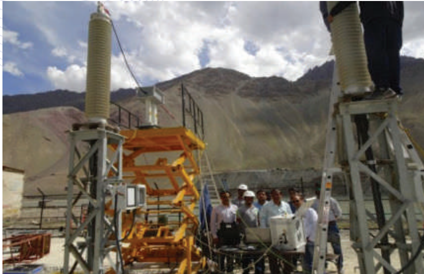
Condition Monitoring Test on 66 kV XLPE Cable, First Time by Diagnostic Testing Team of CPRI, Bangalore at an Altitude of 10000 feet.
