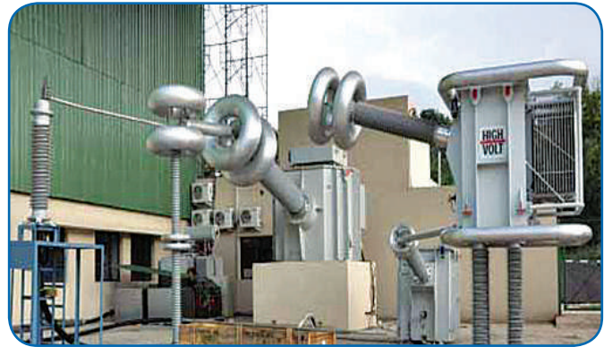
600kV, 4200 kVA Outdoor Transformer
