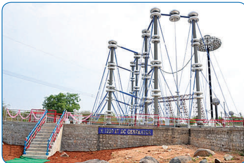
A View of ± 1200 kV DC Test System
