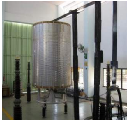
A view of the Line Trap
