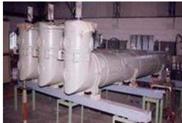
Isolated Phase Bus Duct
