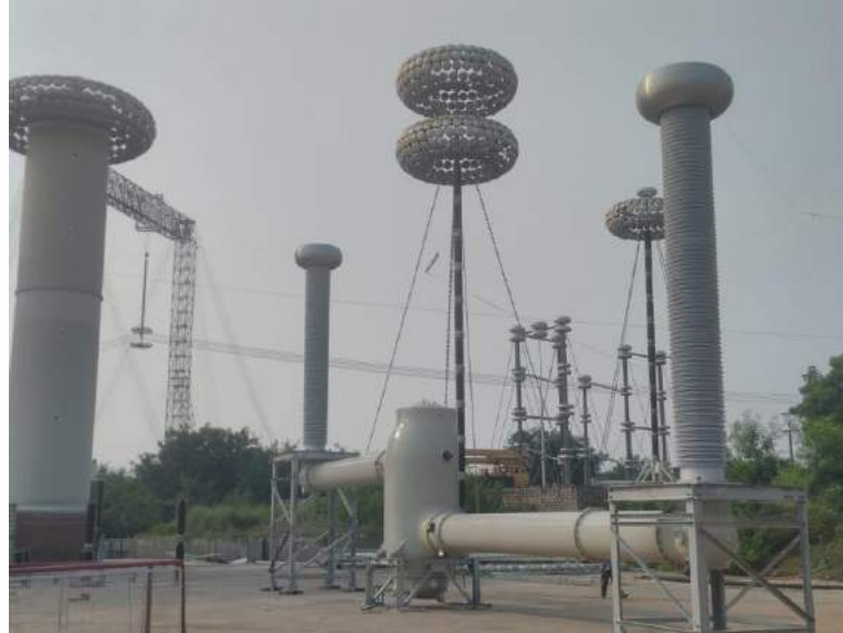
Dielectric tests on 800kV, 5000A, GIS Circuit Breaker
