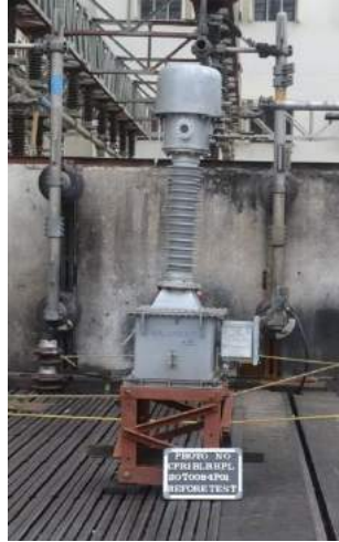
Internal arc test 66kV Voltage Transformer
