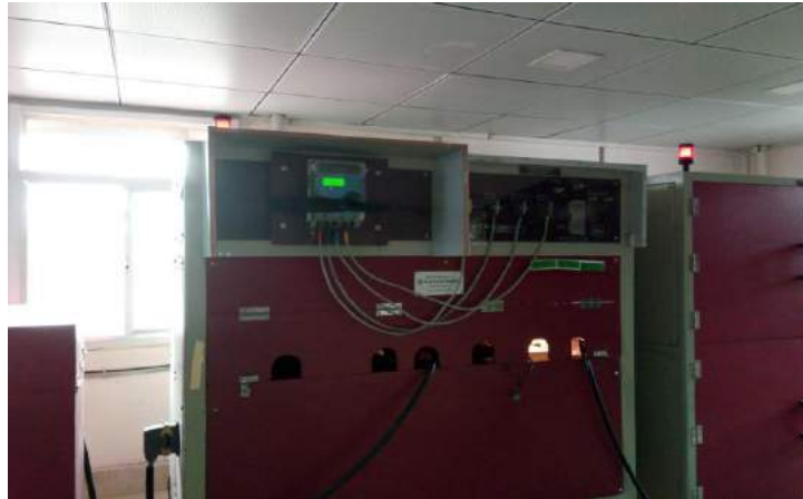
Test of Fault current making capacity and Short time current carrying capacity Test on Smart Meter of UC2 category
