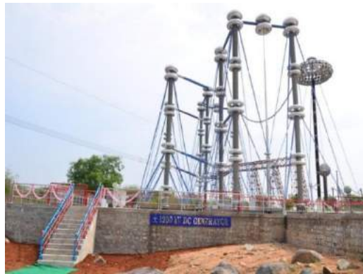
A View of ± 1200 kV DC Test System
