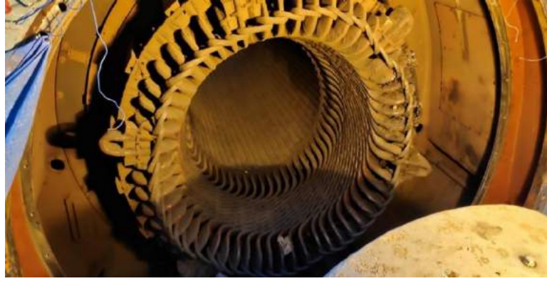
A View of the End Winding from Turbine End
