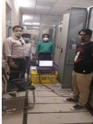
GPS Synchronized End-To-End testing of Distance Protection Schemes
