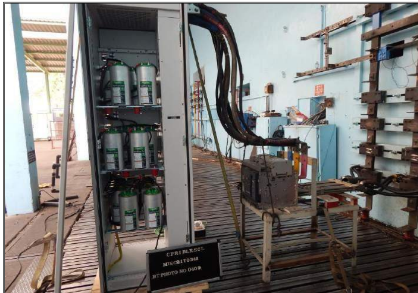
Conditional Short-Circuit test at 415V 65kArms on 415V 534kVAR APFC Panel
