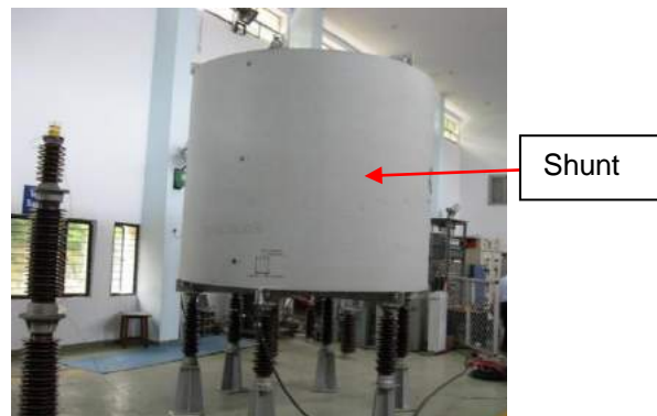
A view of the air core shunt reactor
