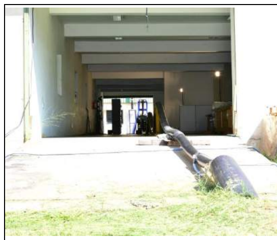
Cable entering in to soil from tunnel
